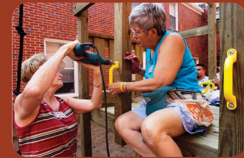
Volunteers work on installation of a playground after it suffered damage from Hurricane Ivan and Tropical Storm Arlene, Florida, USA. FEMA/Lief Skoogfors
